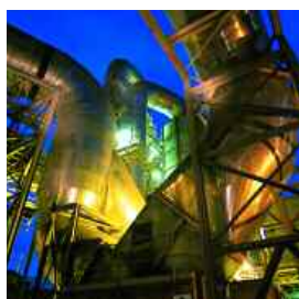
SO 2 emissions can be reduced by the use of modern gas scrubbers
